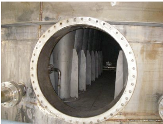
Figure 4: Venturi Tubes shown inside vessel
