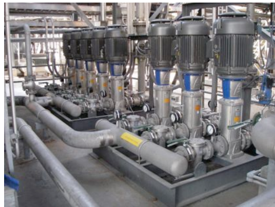
Figure 5: Circulation Pumps installed in one location for maintenance access
