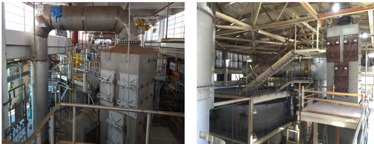
Figure 8. Typical SPC Vessel Installation (Southerly WWTC Left, Mill Creek WWTP Right)
